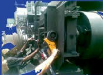
HTW-8D BEING USED ON THE COAL HANDLING UNIT AT JSW BELLARY
