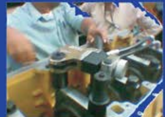
HTW-2L WITH SPECIAL REACTION SOCKET BEING USED ON CATERPILLER ENGINE CRANK SHAFT BOLTS AT HINDUSTAN POWER PLUS, HOSUR
