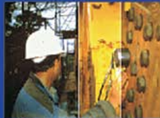
HTW-7D BEING USED FOR BOLT TIGHTENING ON THE LAUNCHING GANTRY USED FOR BRIDGE CONSTRUCTION BY L&T ECC AT BANGALORE
