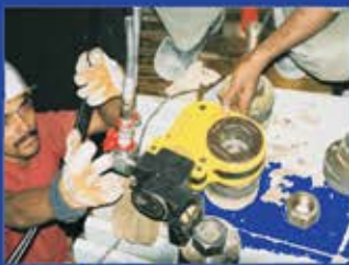
HTW-15S BEING USED ON HYDRO STATOR CORE BOLTS AT BHEL TALA BHUTAN
