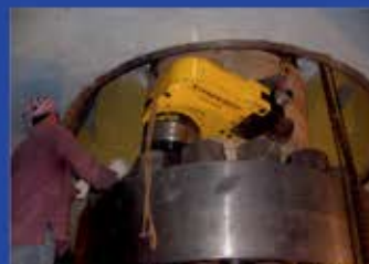
HTW-50S (15000KGM) TORQUE WRENCH USED FOR TIGHTENING TURBINE GENERATOR SHAFT COUPLING BOLT AT NTPC KOLDAM PROJECT.
